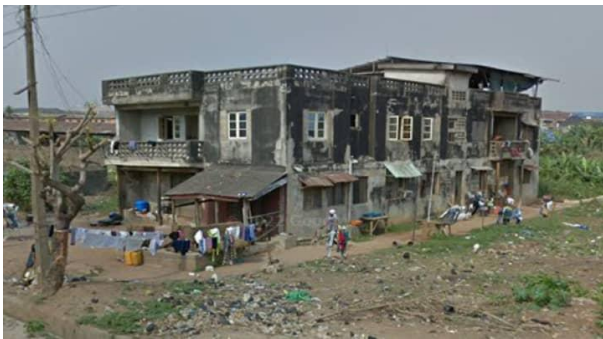
Plate 1. Distressed building at Anibaba Street Street, Oriokuta, Ikorodu North LCDA
